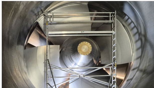
Also the runner blades were inspected as part of the overhaul at the Langkampfen power station.
