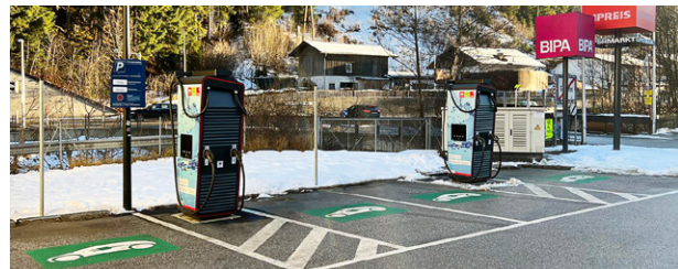
Modern electric charging systems were put into operation at the MPREIS store in Fulpmes.
