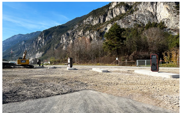
Electric charging stations for the electric trucks were also installed near the construction office in Haiming.
