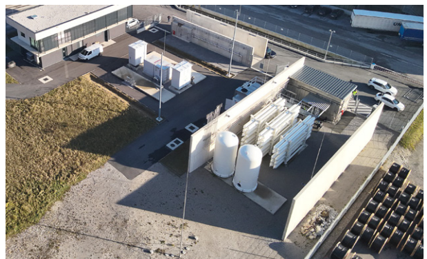
The P2X station in Jenbach
