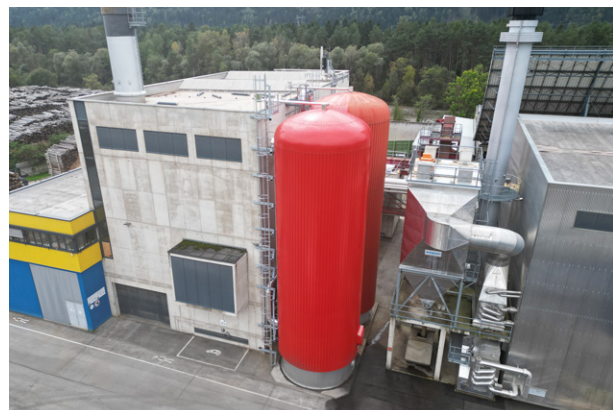
The buffer tank at the Lienz biomass heating plant is being expanded.
