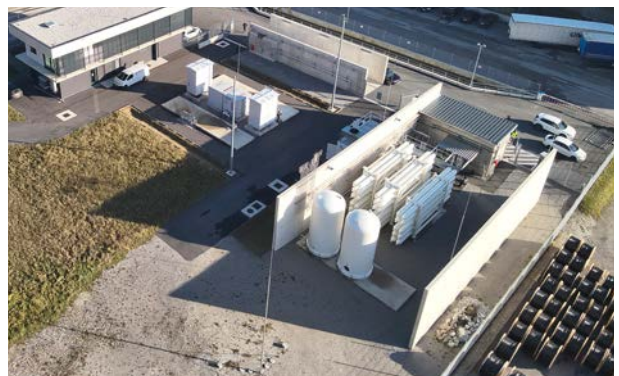
The P2X station in Jenbach
