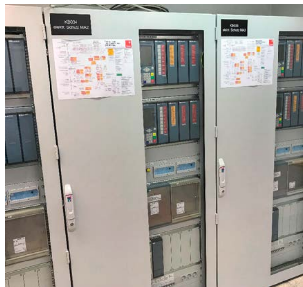
New electrical safety cabinets at Kirchbichl power station
