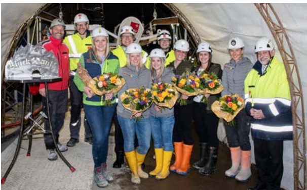
The machine “godmothers” (from left) Aida Osmic, Lisi Lesgi, Elisa Gredler, Sabine Gurgisser, Jaqueline Abfalterer, Anna Edlmair with TIWAG Management Board Members Thomas Gasser (center) and Johann Herdina (right), project manager Klaus Feistmantl (second from right), Johannes Pircher (left), and Christian Schlatter (head of construction management).
