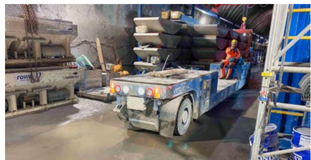
A fully electric construction site train, the VirtuRail, is used for excavation of the diversion tunnel in the Kühtai expansion project.
