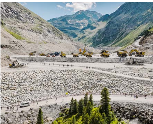
Open construction site day in June 2022: some 6,000 visitors came to look at the Kühtai construction site.
